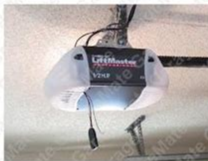
Garage Mate Receiver Installed
